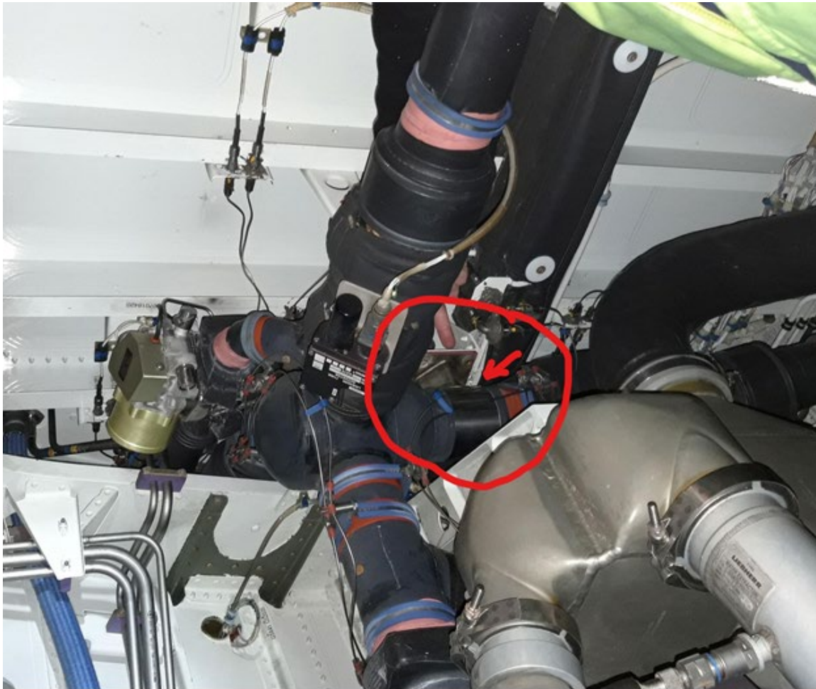
Figure 1: LH bleed air supply duct leak location
