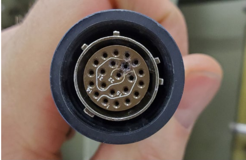
Photo 1 – Electrical connector socket with arcing damage
