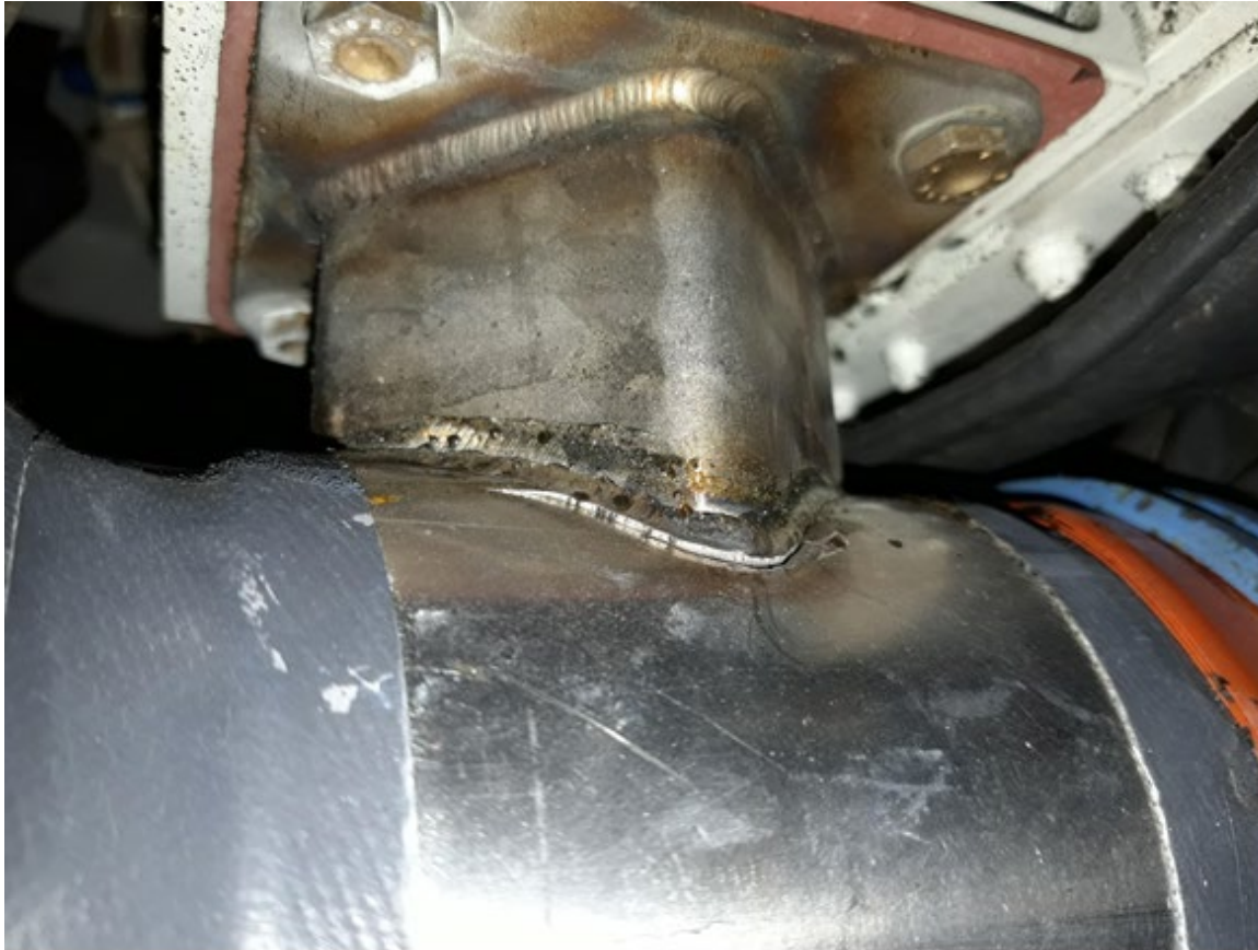
Figure 2: Duct cracked flange shown
