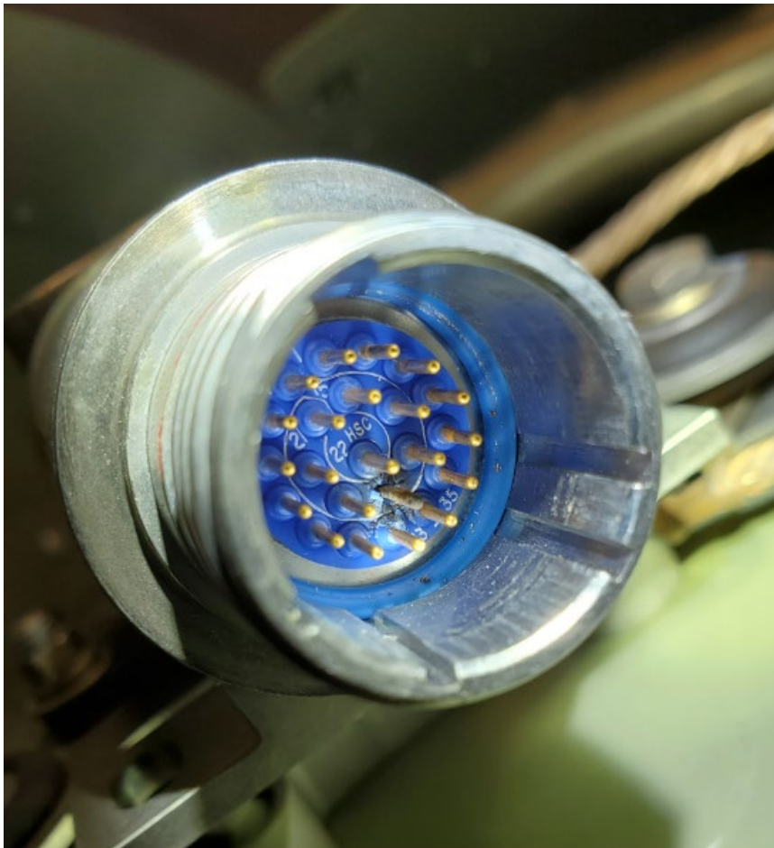
Photo 2 – Electrical connector pin with arcing damage
