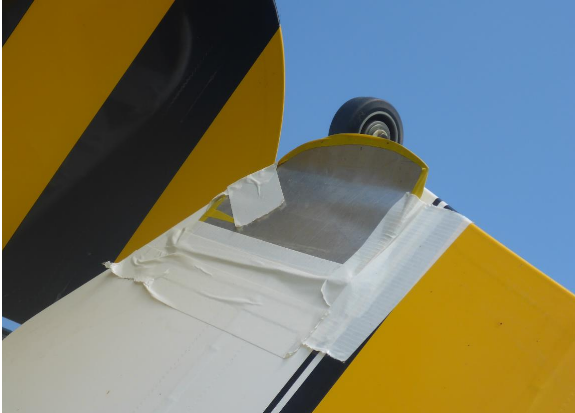
Figure 4. Make-shift elevator trim tab.
